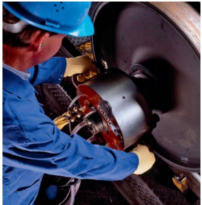
9. Once the set heating time has elapsed, the device automatically switches off. The induction coil is removed together with the bearing inner rings.
