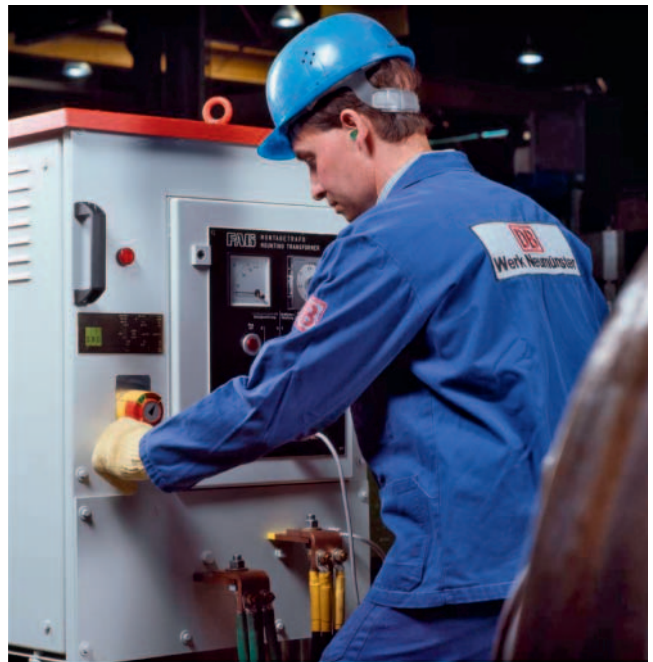
1. The main switch is set to "ON".
