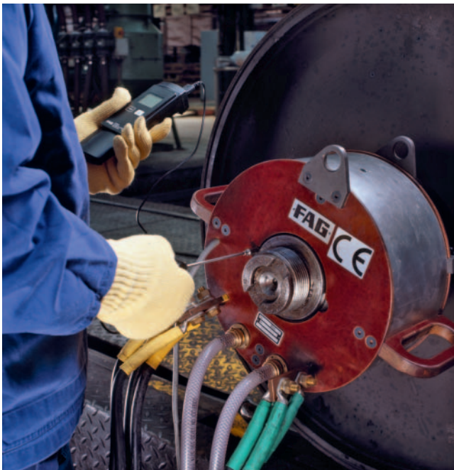
8. During the heating operation, the temperature is measured on the end face of the inner ring.
